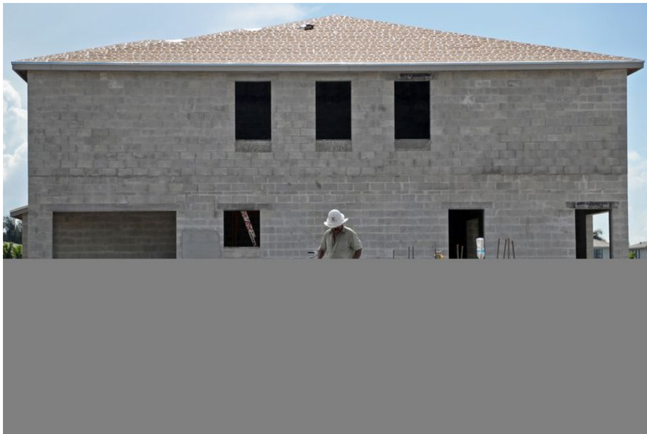
Construction continues on townhomes in the Saddlewood community in Lake Worth Beach on Friday, Aug. 6, 2021. (Amy Beth Bennett / South Florida Sun Sentinel)
