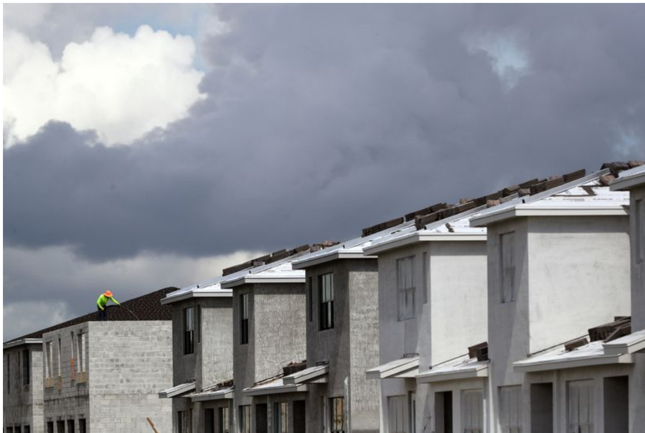
Construction continues on townhomes in the Saddlewood community in Lake Worth Beach on Friday, Aug. 6, 2021. (Amy Beth Bennett / South Florida Sun Sentinel)
