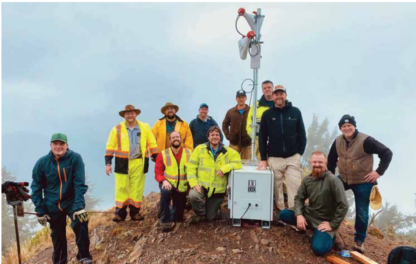
Attorney Damien Hall worked behind the scenes to help the Oregon Internet Response team erect signal towers on hilltops and structures above the McKenzie River Valley east of Eugene. The towers relayed phone and Wi-Fi signals after wildfires cut off service to the area. Photo courtesy of Matt Sayre
